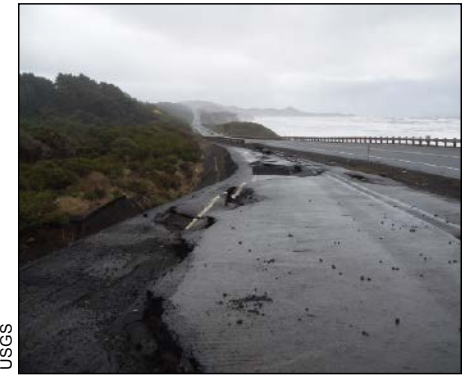
U.S. Highway 101 was moved in 2001 after it was damaged by the Carmell Knoll landslide in Oregon.
