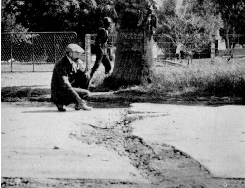
A man examines concrete ruptured by a magnitude 6.7 earthquake on the San Jacinto Fault on 21 April 1918. Credit: Frank Rolfe
