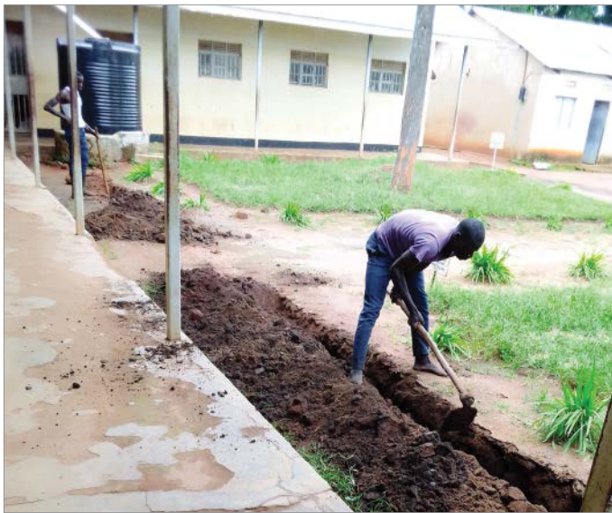
Top: Lightning protection equipment, provided by the African Centres for Lightning and Electromagnetics Network, is installed at the Shone School in Uganda. The school now serves as a model where students, teachers, and parents from other school districts learn about lightning safety. Bottom: A community member digs a trench around the Palabak school in Uganda. The trench will hold a cable attached to conductors running up the building to a lightning rod on the roof. When lightning hits the school, the electricity will be channeled down into the trench to dissipate. Credit: ACLENet
