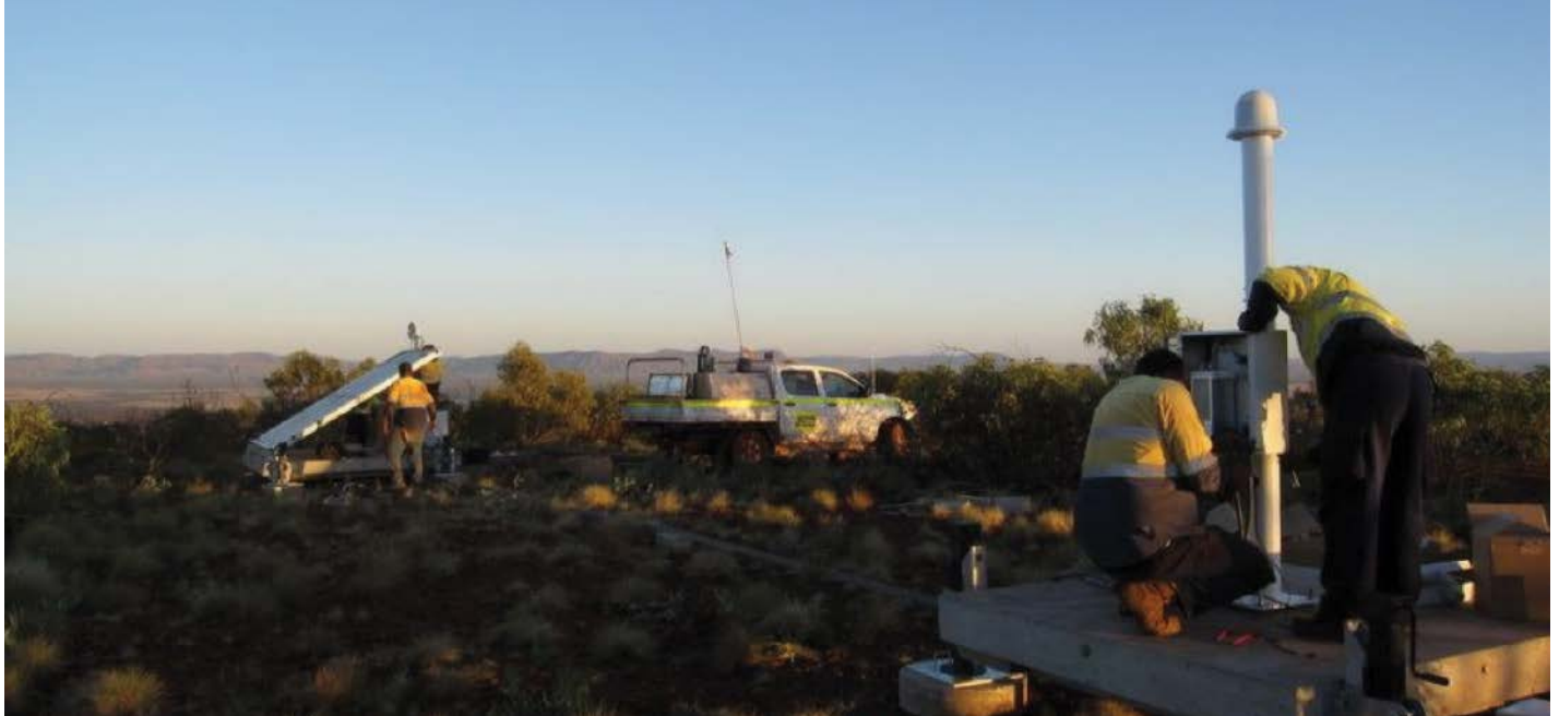
Vaisala engineers install a precision lightning sensor using a solar panel for power in Australia. The sensitive antennas under the white dome detect powerful radio bursts from lightning. The electronics in the enclosure digitize, process, and transmit these signals to a central server in real-time. Credit: Vaisala
