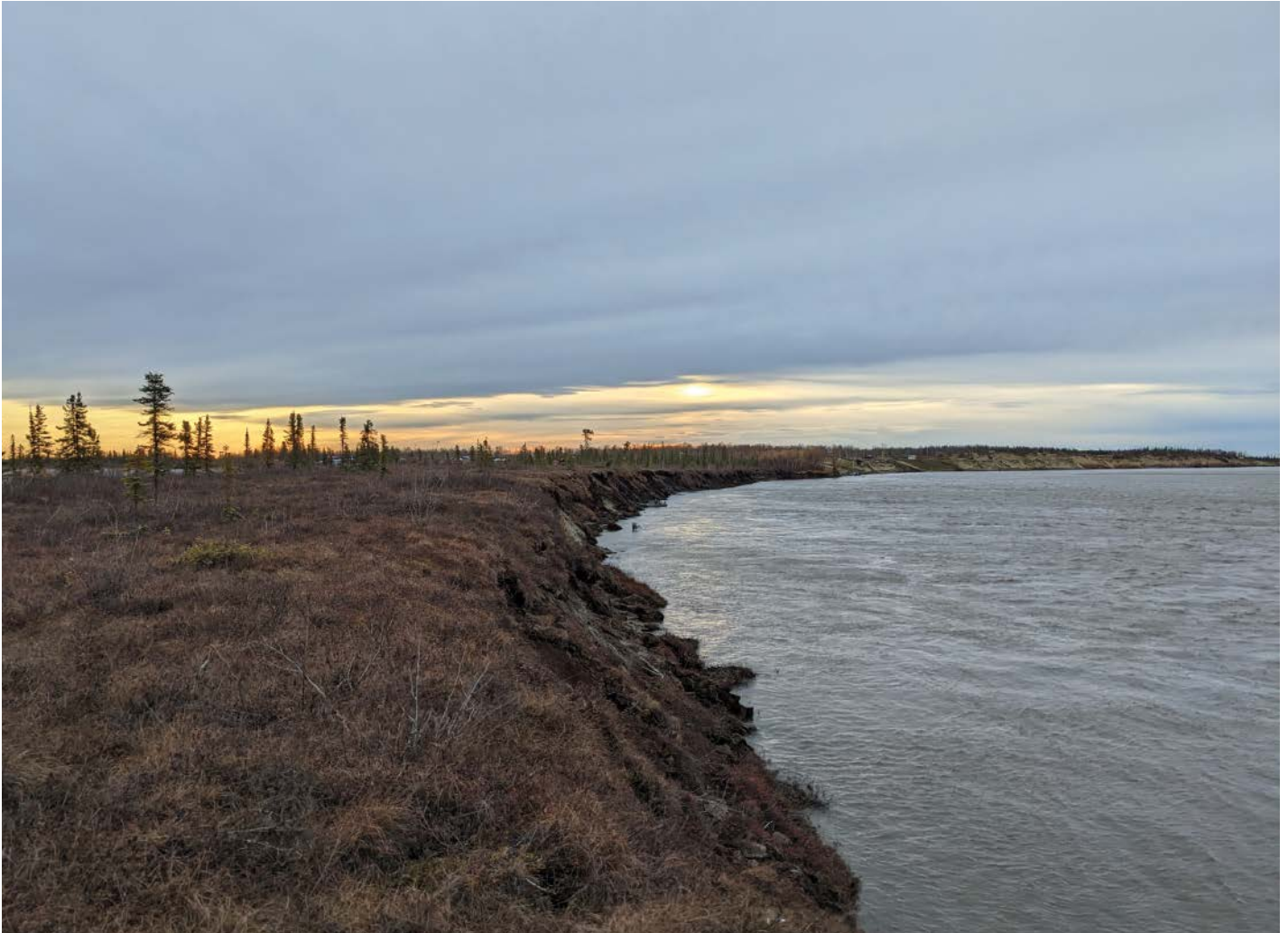
A permafrost riverbank near Huslia, Alaska, exhibits signs of erosion. Credit: Madison Douglas, with thanks to the Huslia Tribal Council for land access
